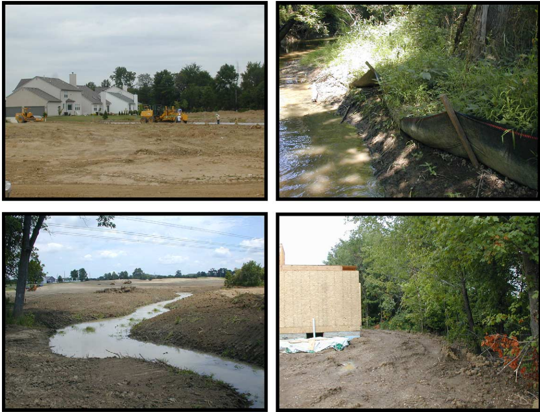
Fig. 8. Construction sites observed during the year 2000 in the rapidly suburbanizing Columbus, Ohio metropolitan area. Upper left, a construction site in the Rocky Fork watershed; the exposed soil is supposed to be stabilized with straw and seeded with grass. Upper right, a properly constructed silt fence retaining sediment on a tributary to Rocky Fork. Lower right, a construction site lacking required soil stabilizing measures and silt fencing is located adjacent to a Big Walnut tributary (the tree line is the stream bank). Lower left, another Big Walnut tributary bulldozed for new construction.
