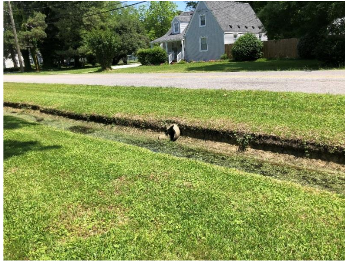
FIGURE 1: EXAMPLE OF OVERDITCHING- STEEP SIDE SLOPES
