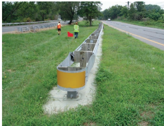
DelDOT is testing various weed control barriers for use under guard rail
