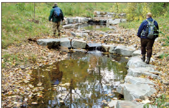
Step pools, such as this one installed along Stony Run in Baltimore, Maryland, consist of a series of low elevation pools and weirs and are designed to dissipate energy along stream reaches that are downcutting.
