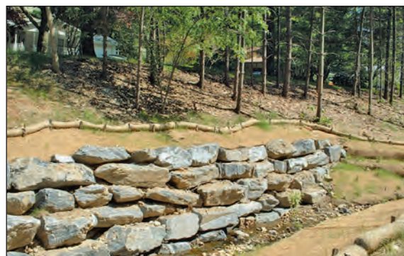
The boulder revetment provides a more structural and immediate method to stabilize the stream bank in this Howard County, Maryland, stream reach.
