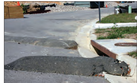
Asphalt barriers are used to direct stormwater runoff away from an inlet and into a sediment basin.
