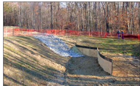
Sediment basins collect construction site runoff and associated sediment, preventing it from entering nearby streams.
