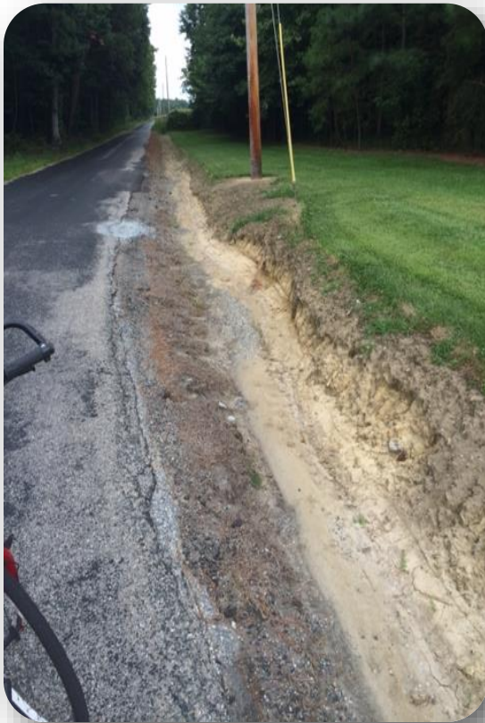
Figure 38 Ditch after Improper Cleaning Image Credit: Roger Bollman
