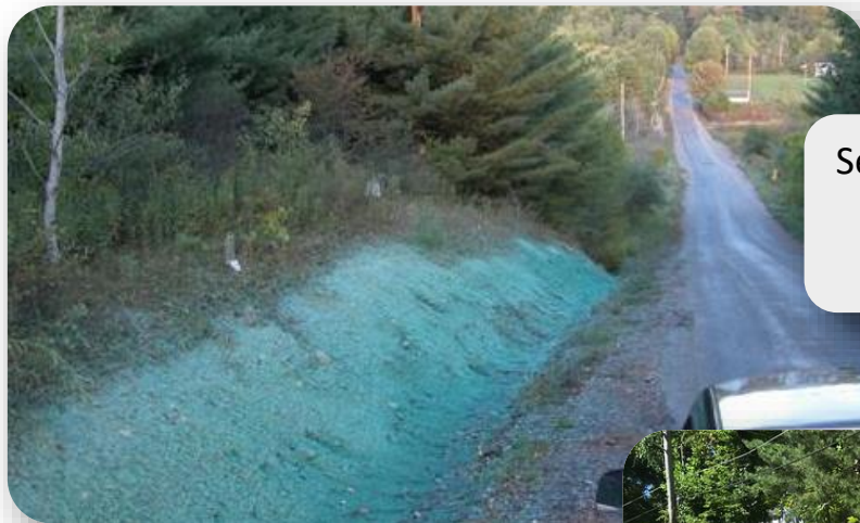
Figure 8: Ditch with Hydroseed Image Credit: Cornell University http://ei.cornell.edu/watersheds/Ditches/Ditch_7.html
