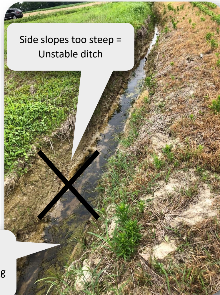
Figure 41: Unstable Ditch Geometry with Steep Side Slopes
