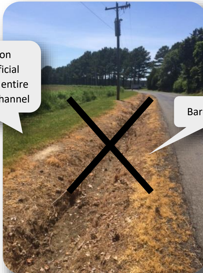
Figure 31: Ditch with Herbicide Damage Image Credit: Roger Bollman
