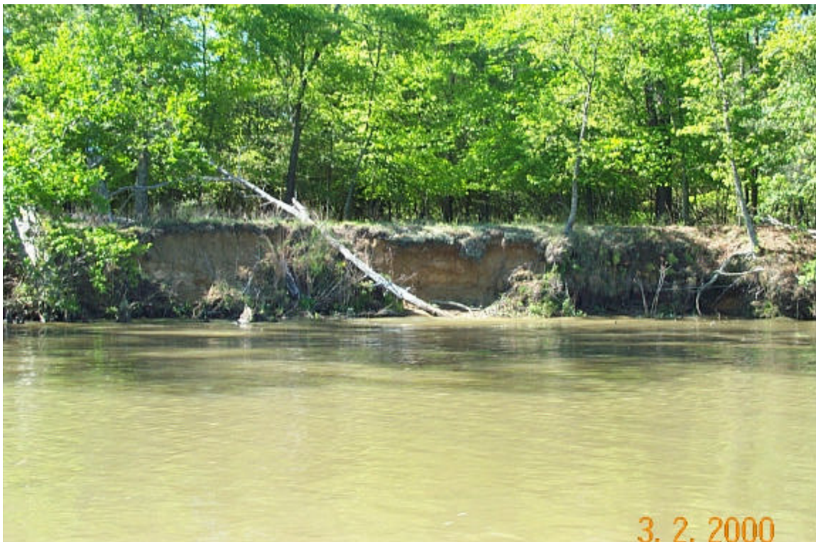
Figure 3-5. Shoreline erosion along Wright’s Island
