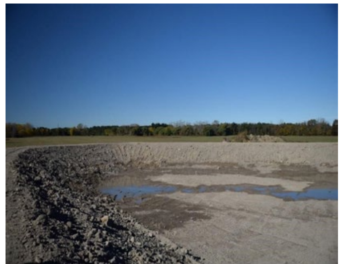
Figure 5: Pond volume is calculated from the irrigated area and depth of irrigation needed. This irrigation pond in Michigan is about 20 feet deep.
