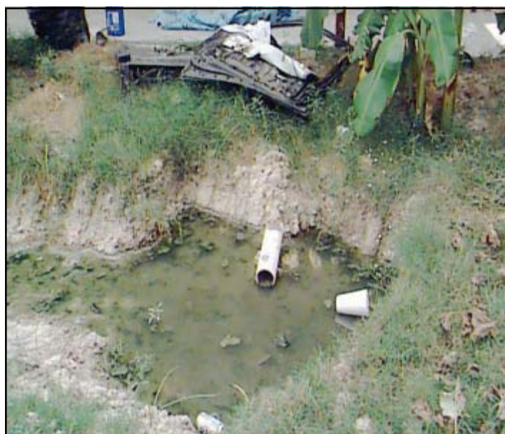
Figure 2. An Example of Hydraulic Failure (Houston/Galveston Area Council, 2000)
