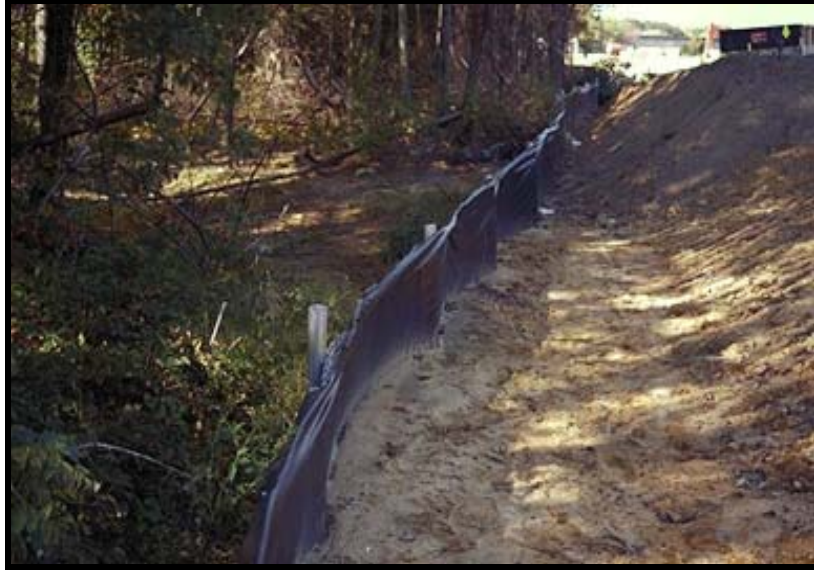
Figure 13. Silt fence used as perimeter control to protect wetland (Photo source: MDE, no date)
