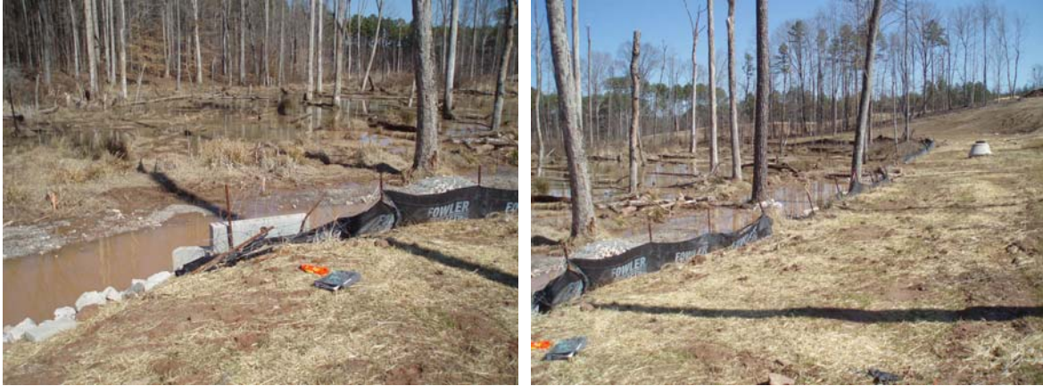
Figure 18. While some impacts to this wetland in the Neuse River Basin, NC were permitted, the local regulations require proper erosion and sediment controls to protect streams and wetlands from excessive sedimentation. The silt fence shown in these photos has not been properly maintained and allows discharges of sediment into the stream and wetland. Better enforcement and inspections might have prevented this situation.
