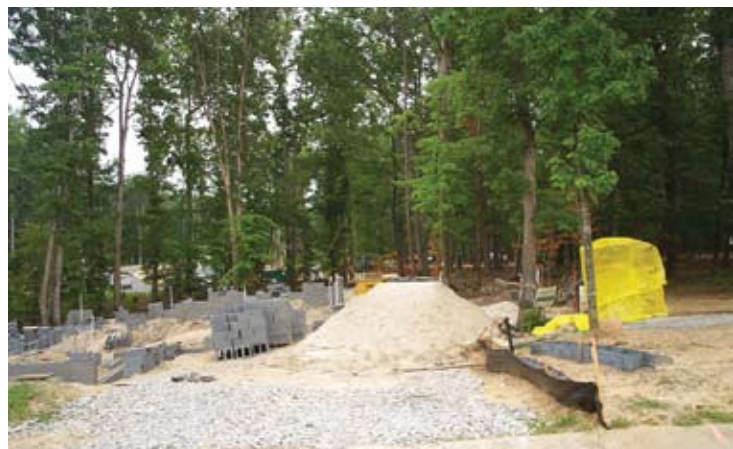
Figure 6. Improper disposal of construction materials and inadequate protection negatively impact trees at a construction site.
