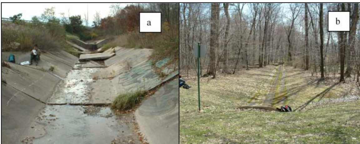
Figure 39: Restoration of Channelized Stream Segments Candidate site for structural repair (Panel A) and natural channel restoration (Panel B).
