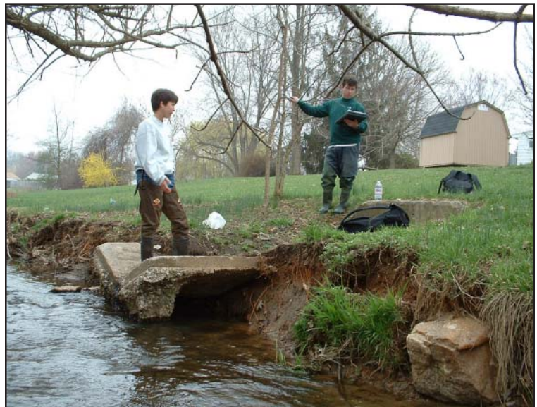
Figure 3: Site Impact Assessment at Outfall and Bank Erosion Location
