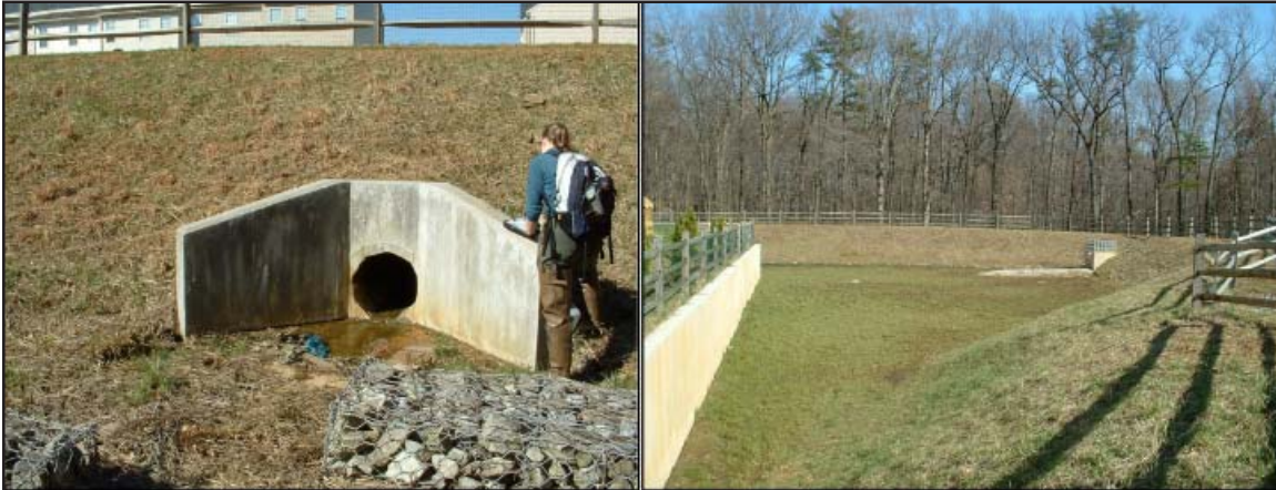
Figure 18: Investigate Existing Storm Water Treatment Practices When assessing an outfall, you may want to take a quick trip up-pipe to determine if the discharge is controlled by a storm water facility. In this case, the outfall is the discharge point for a dry pond. Dry ponds do little for water quality and are therefore good retrofit candidates.
