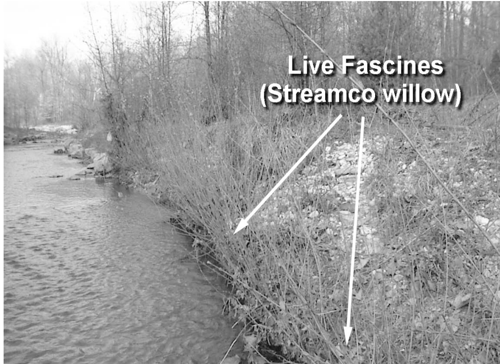
Photo 4.32: Live fascine installation along streambank toe with excellent branch sprouting (Streamco willow).
