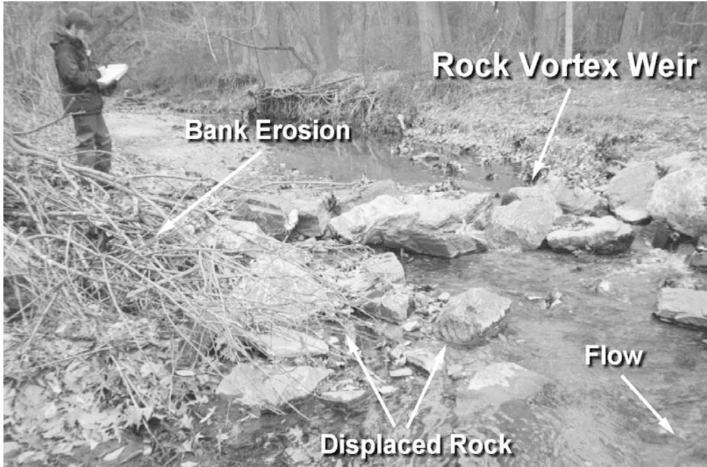
Photo 5.7: Reduction in channel cross section at this rock vortex weir caused channel widening and practice failure.
