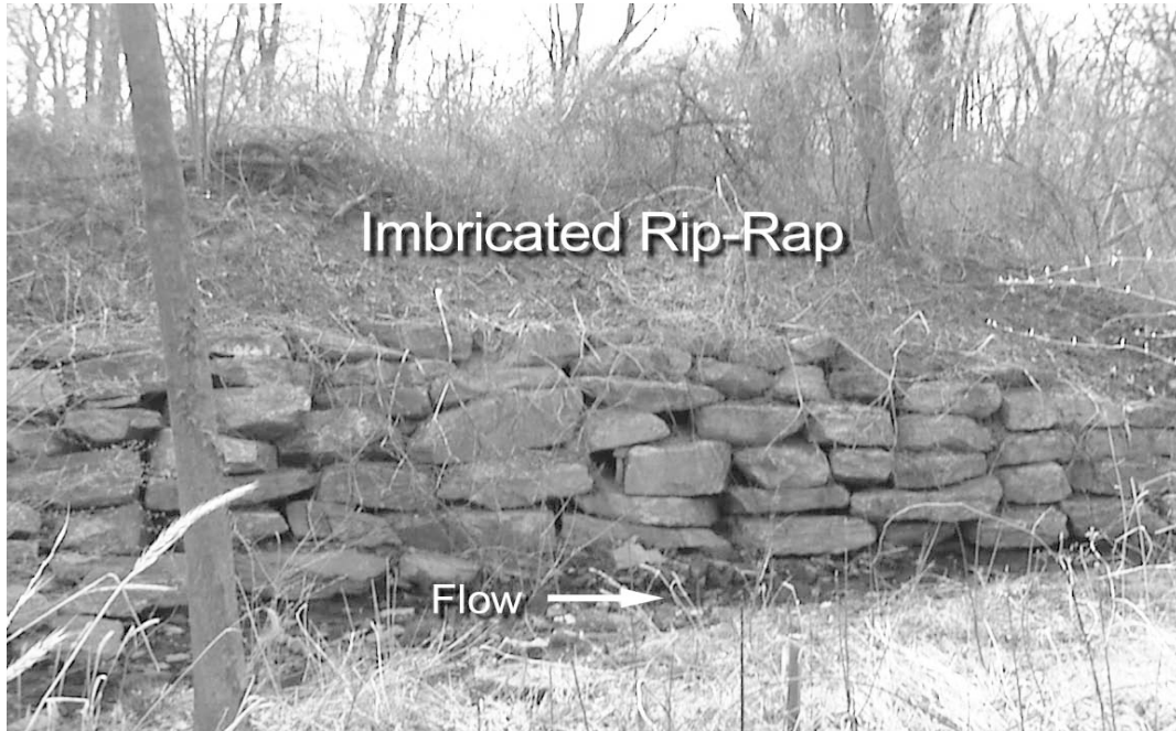
Photo 4.5: Imbricated rip-rap revetment protecting 15 foot tall unstable streambank. A parking lot lies at the top of slope.
