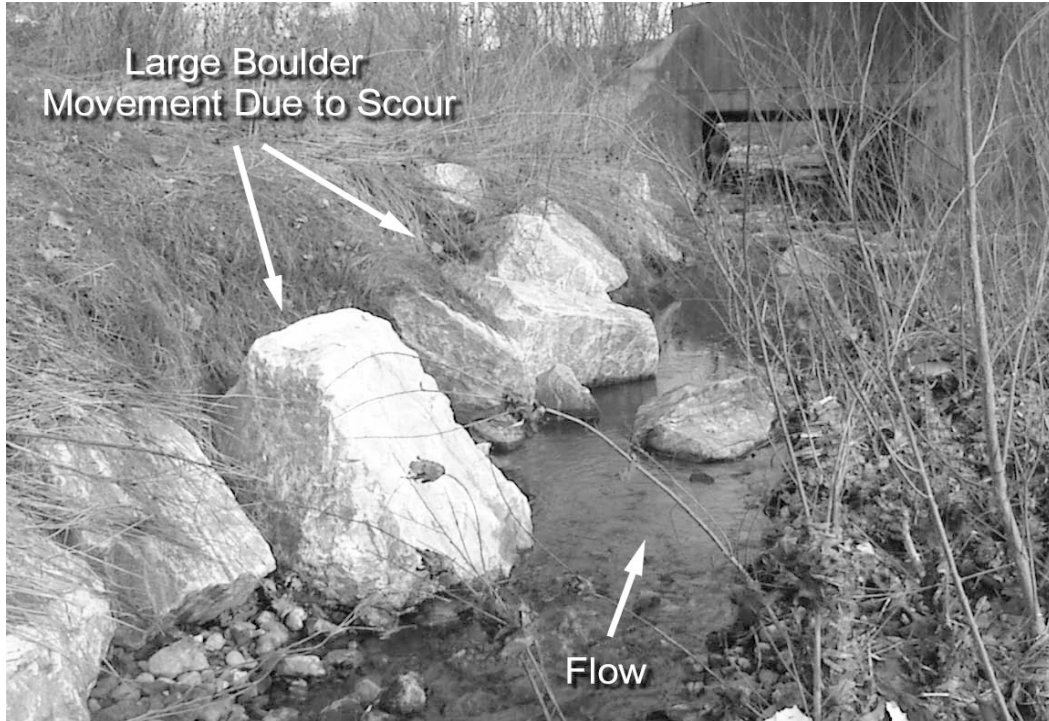
Photo 4.6: Large boulder revetment that has experienced scouring along the toe of the streambank and movement of practice materials.
