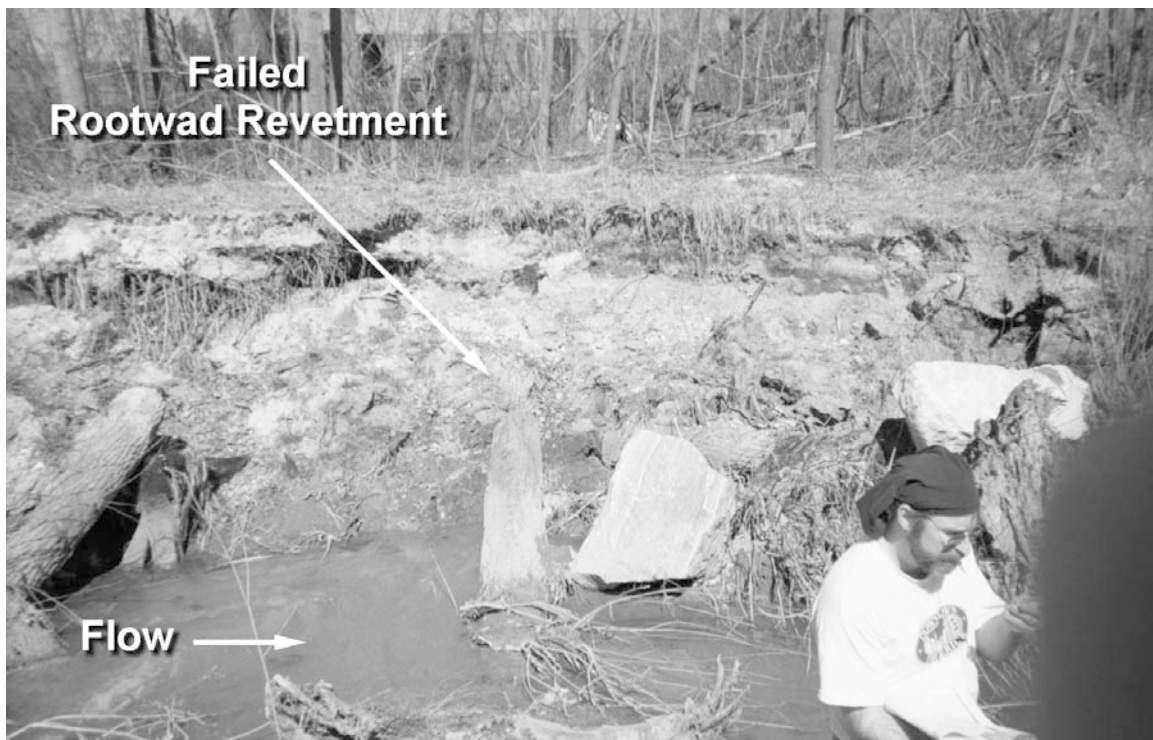
Photo 5.1: Rootwad failure due to incorrect meander geometry. Meander radius was too small for existing stream conditions.
