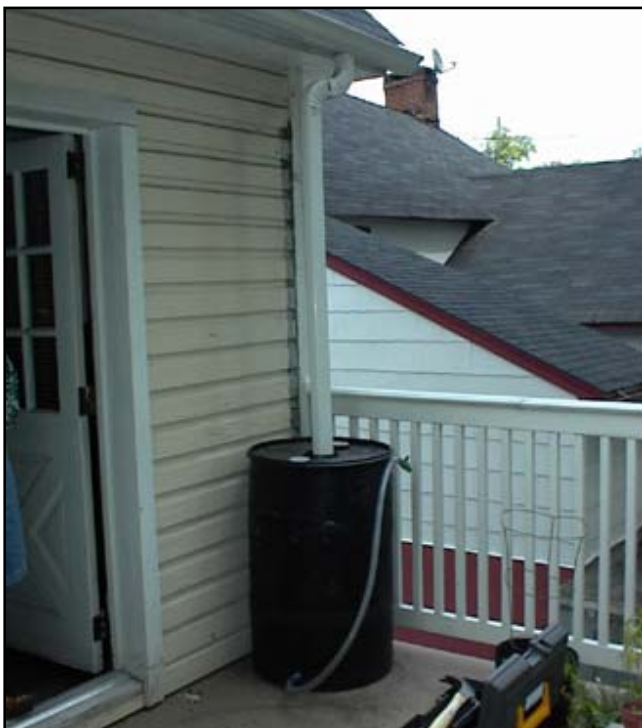
Figure 2: Rain barrel installed on a balcony due to space constraints on a small lot. C
