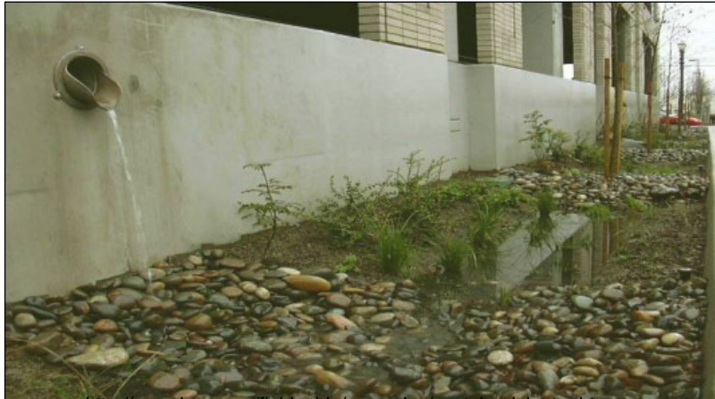
Figure 5. 55 This flow-through planter collects runoff from the rooftop of a parking garage and is incorporated into the structure
