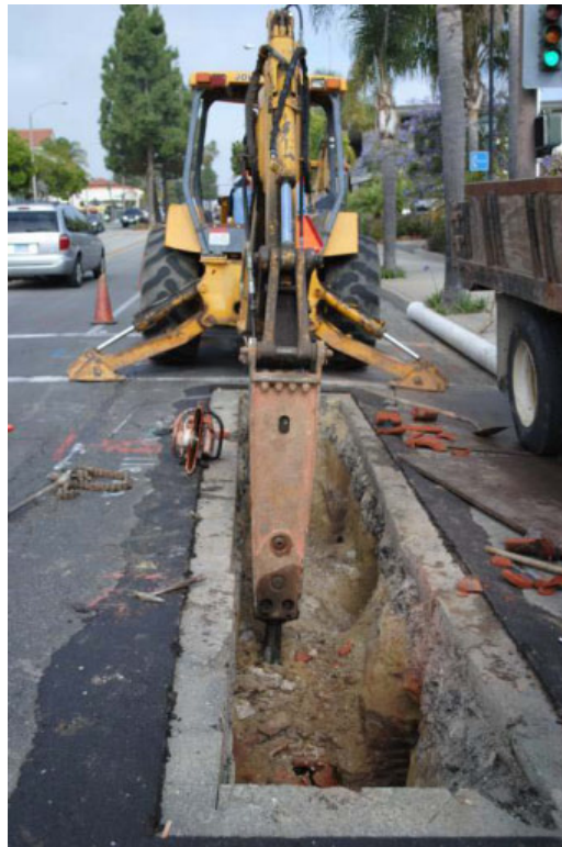
Figure 5-1. Repair of Leaking Sanitary Sewer and Storm Drain Detected with Canine Tracking.
