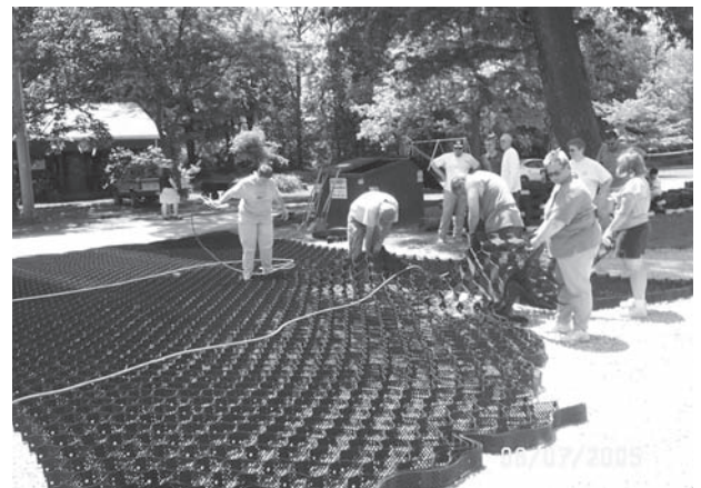
Geoweb installed at Legion Park. Geoweb is a plastic-like and honeycomb shaped cellular confinement system that is manufactured by Presto Company.
