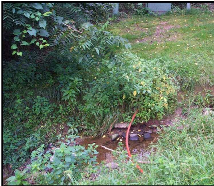
Figure 38. - Exposed electric wires at a Paxton Crossing stream
