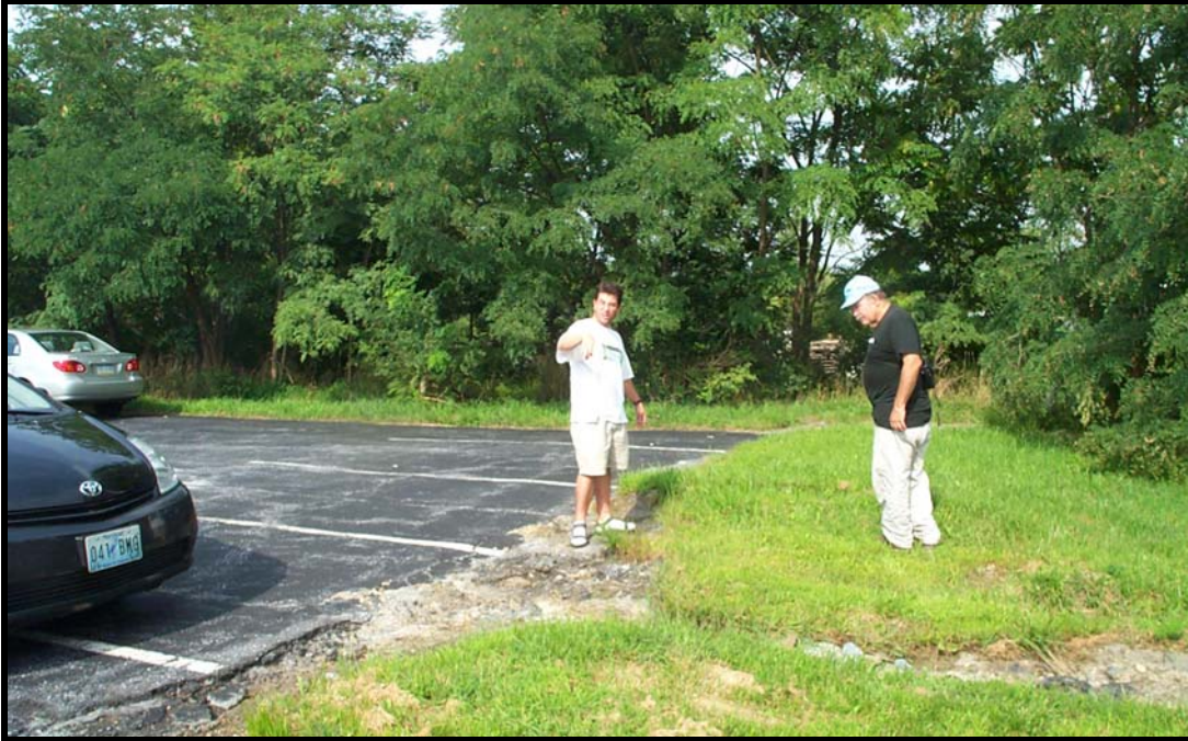
Figure 27. Runoff from Vartan Property office building parking lot causes channel erosion just upstream of Davis Landscaping
