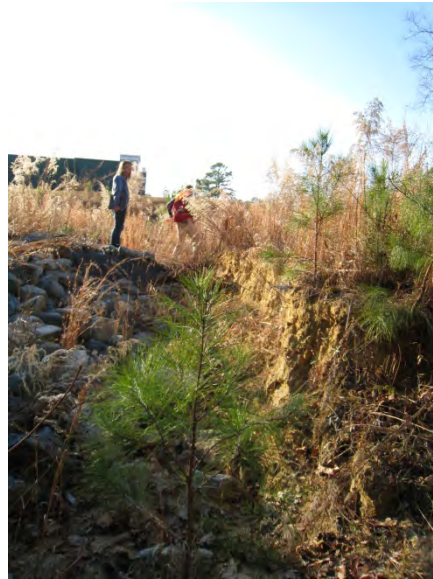
Figure 2: Dam section eroded out at spillway
