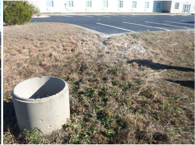
Figure 2: Riser structure at northern end of basin
