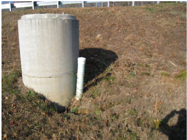
Figure 4. Basin outlet, with erosion at base
