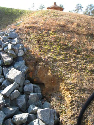
Figure 5. Steep basin inlet, eroding
