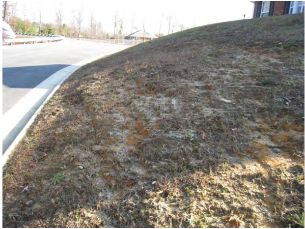
Figure 2. Bare, sandy soil on slopes
