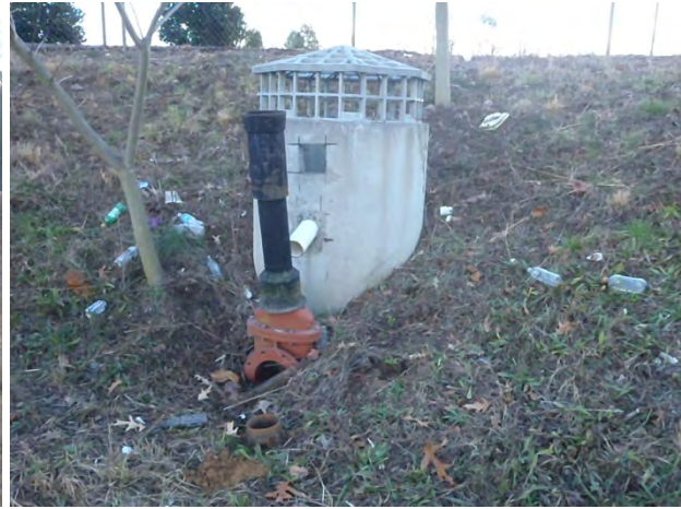
Figure 2: Trash around outlet structure
