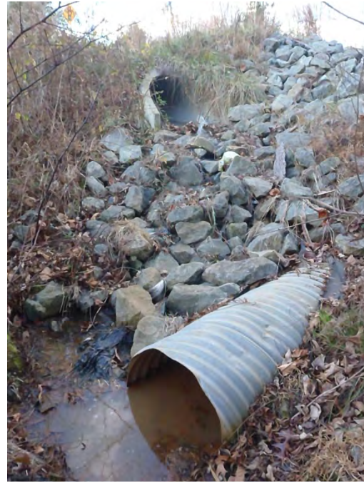
Figure 2: Metal outlet pipe partially clogged
