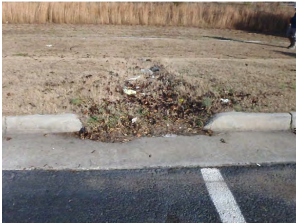
Figure 3: Partially clogged inlet to basin
