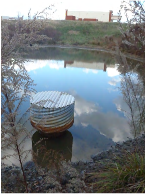
Figure 1: Wet pond with metal overflow structure
