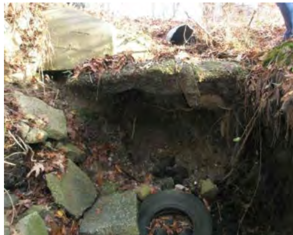
Figure 1: Outfall (end section, upper left)
