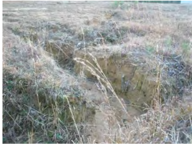
Figure 2: Erosion of outlet
