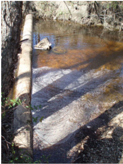
Figure 27C: Reach OTC-2, UT-1: The exposed utility pipe crosses the stream and is cracked.
