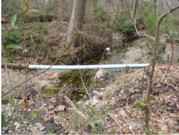
Project 23: Vulnerable sewer line (OTC-4, MI-1)
