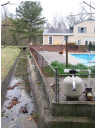
Figure 24G: There is a potential Illicit discharge of residential swimming pool discharge connected to storm drain system located at the end of Old Town Drive.
