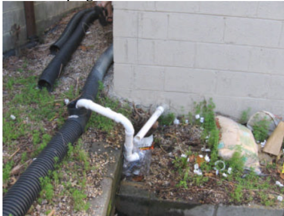
Project 1a. Downspouts from businesses on Route 1.
