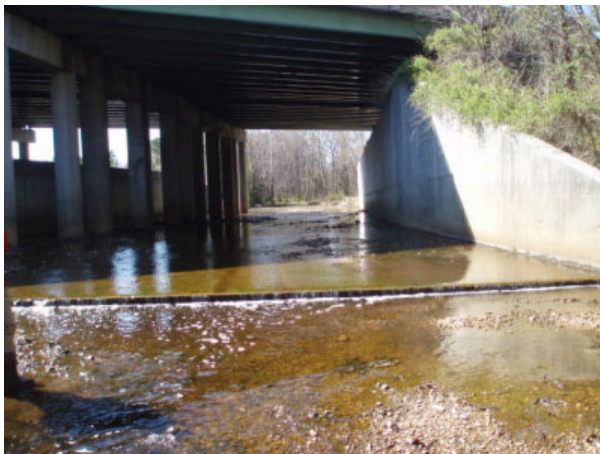
Project 12B: Drop and shallow flow creating a fish barrier (OTC-2, SC-1)
