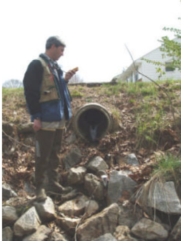
Project 24C: Reach TB-07, OT-1: Concrete outfall that is chipped and cracked.
