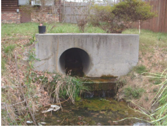
Figure 24F: Reach BB-03, OT-1: Concrete pipe that drains a residential neighborhood.
