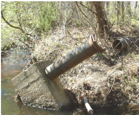
Project 29: Reach BL-03, OT-1 metal pipe that has section broken off.
