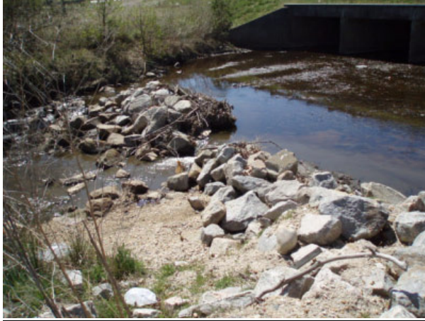
Project 12A: Rip rap creating a fish barrier (OTC-1, CM-1)
