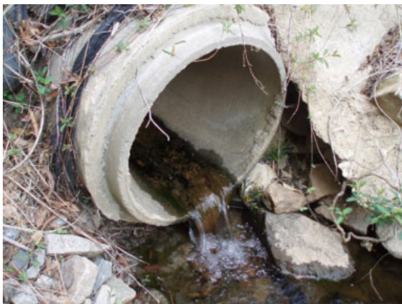
Project 24B: Reach OTC-3, OT-1: Outfall with strong odor and pool quality issues
