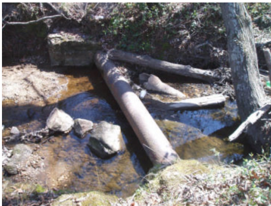
Figure 27D: Reach TB-01, UT-01: The pipe is corroding and cracking. There is orange iron bacteria associated with the pipe. The pipe appears to be out of service and could be removed.
