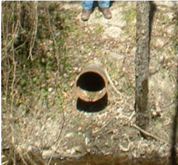
Project 24D: Reach BL-03, OT-2: Metal pipe located behind the Lakeview Elementary School.
