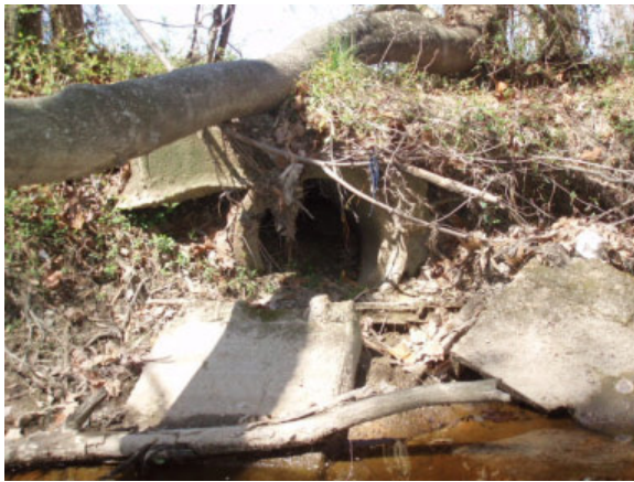
Project 24A: Reach OTC-1, OT-2: Outfall with suspicious pool quality
