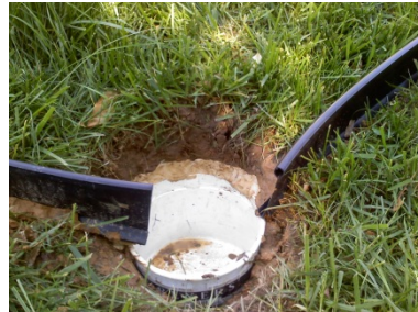
Runoff collection bucket with lawn edging.
