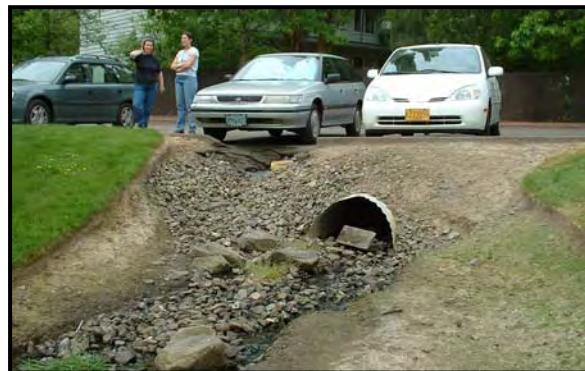
Figure B.21: Example of where culvert repair may be needed in combination with buffer planting and storm water control.
