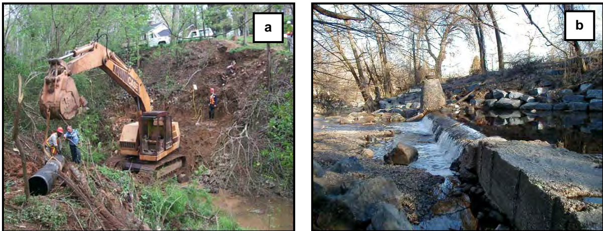
Figure B.19: Structural repair or relocation of sewer lines may be necessary to stop leaking pipes as shown here (panel a), or to restore fish passage at potential fish barriers like the one shown here (panel b).
