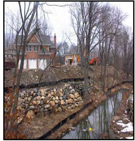
Figure 2.9: Loss of Stream Buffer
