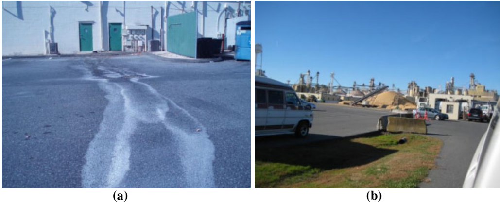
Figure 4.27. (a) Staining on parking lot leading to storm drain at Hunan Delight (HSI_5) and (b) Raw materials stored outside without cover at the Perdue plant (HSI_12).
