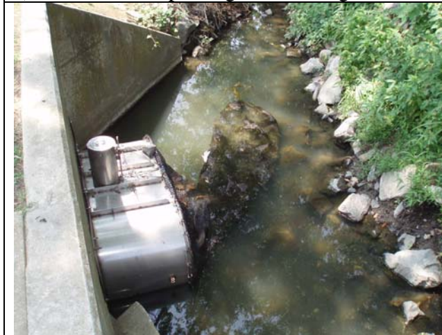
b) Glenwood Elliptical outfall is 54 inch.
