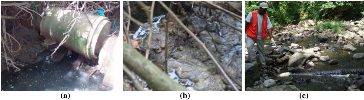
Figure 8. (a) WR702: Sanitary leakage into Western Run traced upstream to one of two private units. (b-c) WR256: Sanitary line broken in two locations behind residential townhome development.
