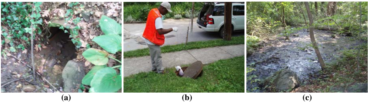
Figure 9. (a-b) WR254: Dye testing revealed infiltration from a sanitary line into the storm drain system in an outfall behind a residential home. (c) Sanitary seepage from a hillside has not been successfully traced in an adjacent neighborhood.
