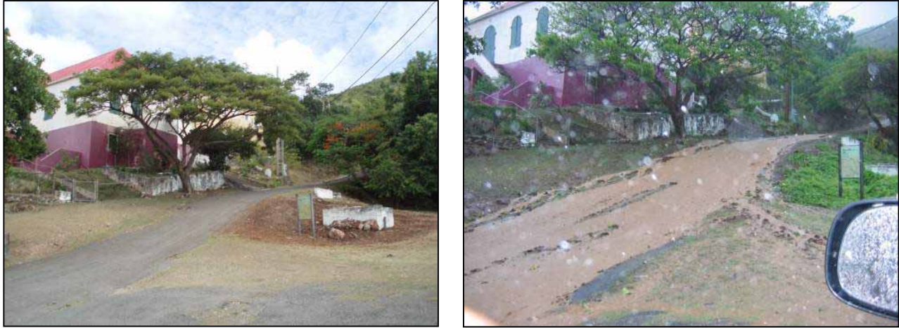
Figure 7. Johnny Horn Rd before (left) and during a rain event (right, photo courtesy of CBCC).
