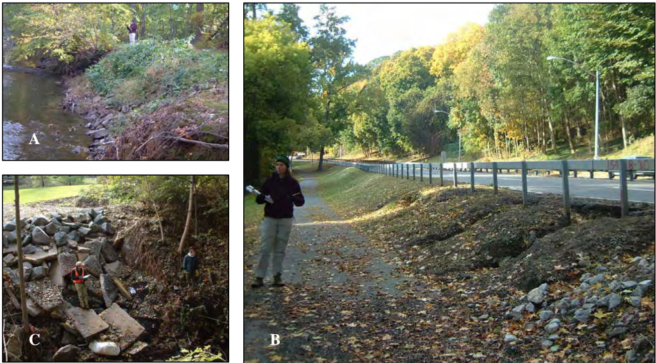
Figure 3-6: Problems with (A) stream bank erosion, (B) erosion in the upland corridor, and (C) head cuts were noted by field crews. These examples are from reaches in Bronx River Upper Direct Drainage (BRU-6 and BRU-5) and Manhattan Park Brook (MP-3), respectively.
