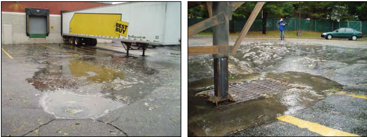
Figure 3-8: A sewer overflow was observed in the loading area in back of the Best Buy shopping center on Central Avenue in Fulton Brook Subwatershed (site ID FB-H2). Overflow drained into storm drain, which discharged directly into stream.
