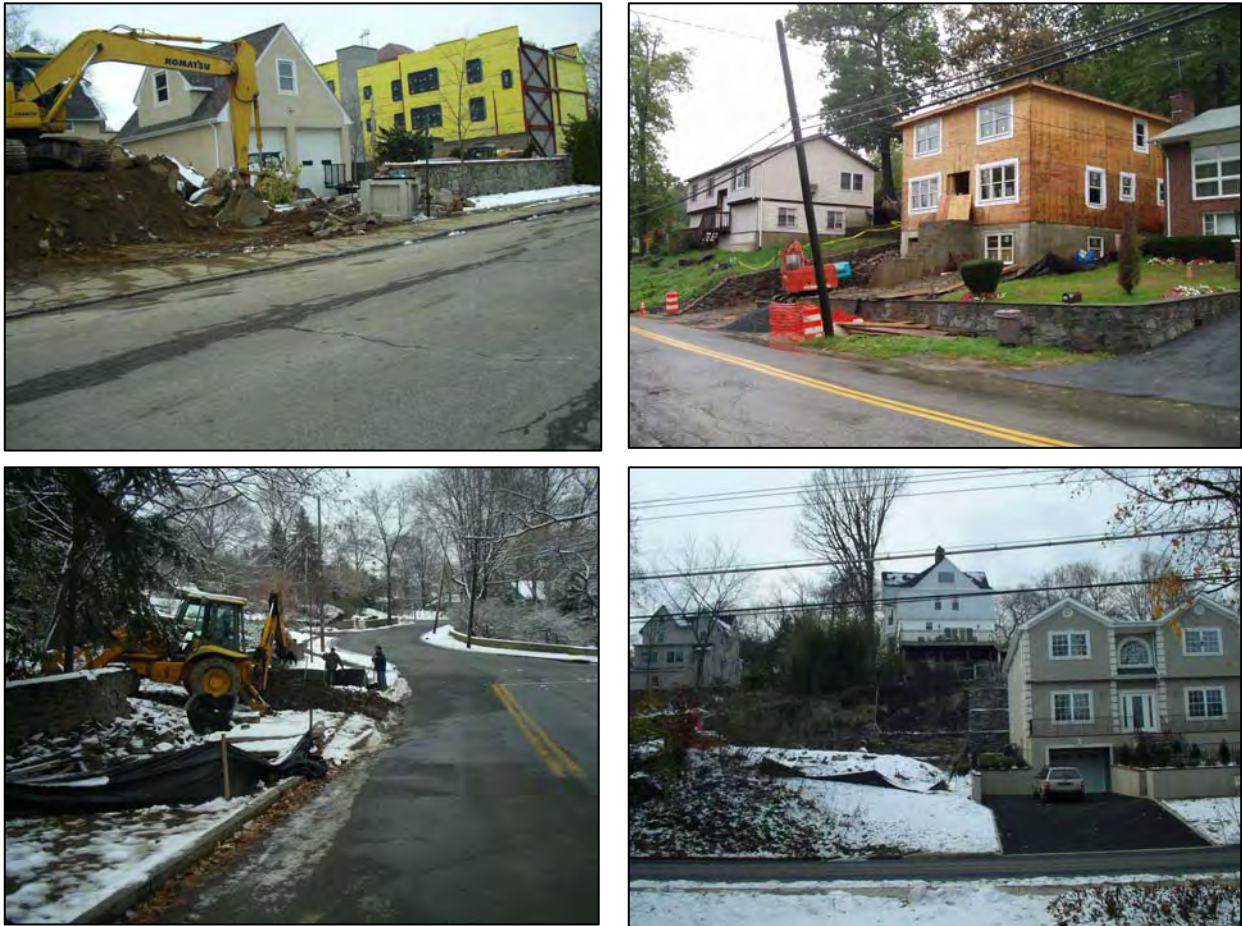
Figure 3-18: Construction in residential areas was mostly single lot infill and redevelopment with poor erosion and sediment control implementation.
