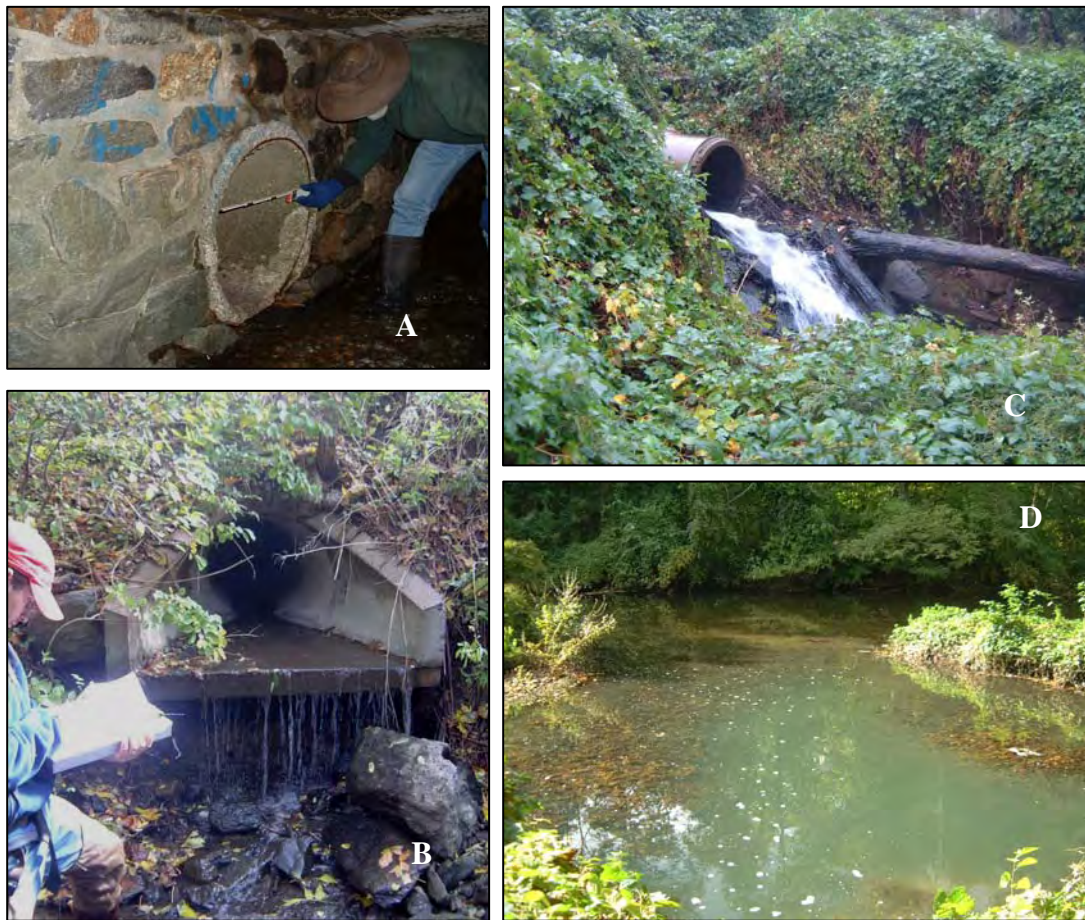
Figure 3-3: Field crews evaluated outfalls (A), looking for maintenance issues like undercutting (B) in Sprain Brook at reach SB-21 and suspected illicit discharges for further investigation like OT-1 discharge in Sprain Brook at reach SB-6 (C) and as evident with suds and murky/greenish discharge in Bronx River Middle Direct Drainage at reach BRM-1a (D).
