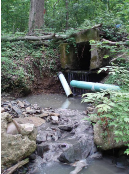
Figure 3.5. Sewage discharges that originate from the sanitary sewer, such as this broken pipe, are classified as sanitary sewer overflows in Baltimore City and are the responsibility of the Wastewater Engineering and Maintenance Program (Source: Center for Watershed Protection).
