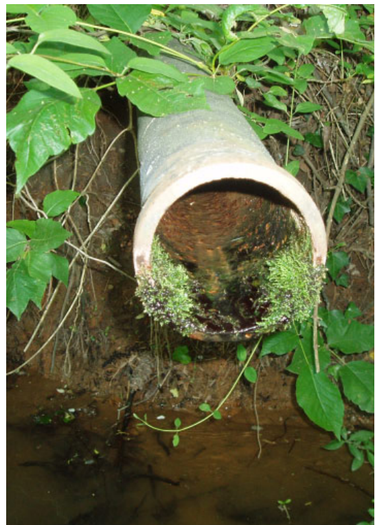
Figure 3.1. Illicit discharges are defined by EPA as any pollutant discharge to the storm drain system that is not permitted. Vegetative growth on this
