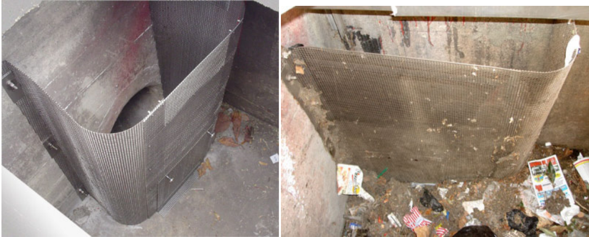
Figure 4.6. Catch basin inserts can remove 100 percent of trash from contributing drainage areas (Source: City of Los Angeles Stormwater Program http://www.lastormwater.org/siteorg/program/poll_abate/cbscreens.htm )
