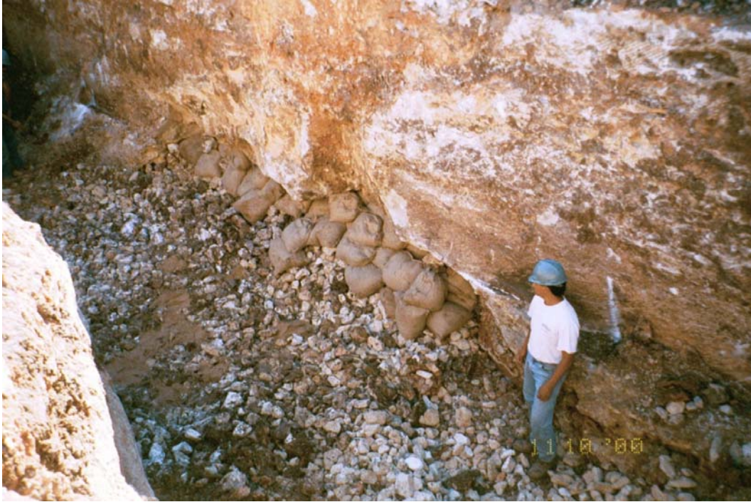
Sand bags placed inside cave opening.
