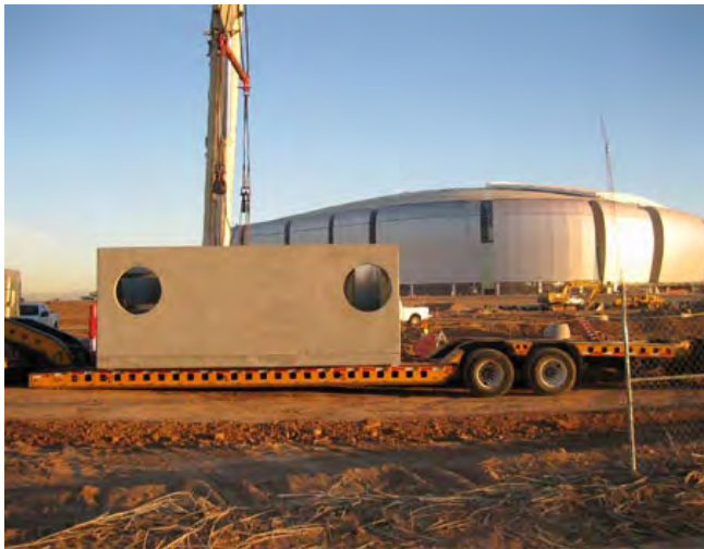
Thirteen subsurface swirl separators manage the first flush of stormwater at the Arizona Cardinals Football Stadium, a 120 acre site that is mostly impervious. Photo: Civil and Structural Engineering Magazine
