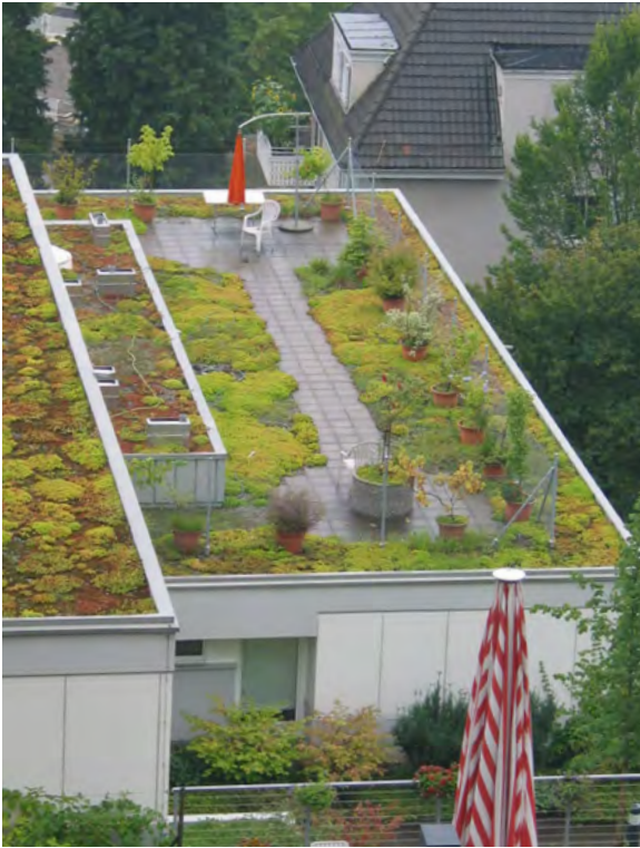
Intensive vegetated roofs can provide usable open space in addition to their stormwater management function. Photo: Rosey Jencks
