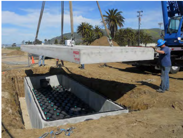
Media filter installation. Photo: Storm Water Solutions
