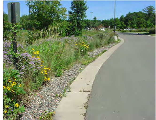
An infiltration trench along a roadway in Lino Lakes, MN. Photo: Minnesota Pollution Control Agency
