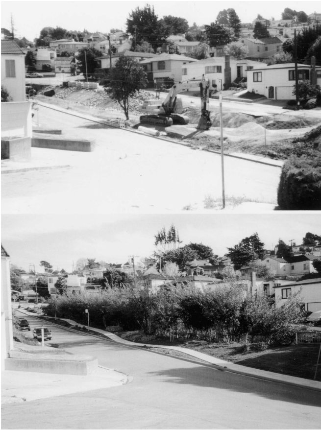
Figure 1. Photographs of the site during restoration in 1996 (top) and after restoration in 1998 (bottom). (Photographs by Lisa Owens-Viani.)
