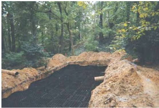
Subsurface Infiltration Bed using Rainstore™ blocks for storage media, Washington National Cathedral, DC
