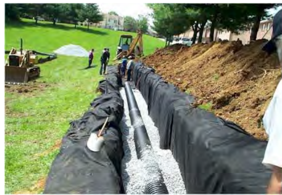
Infiltration trench Chester County, PA
