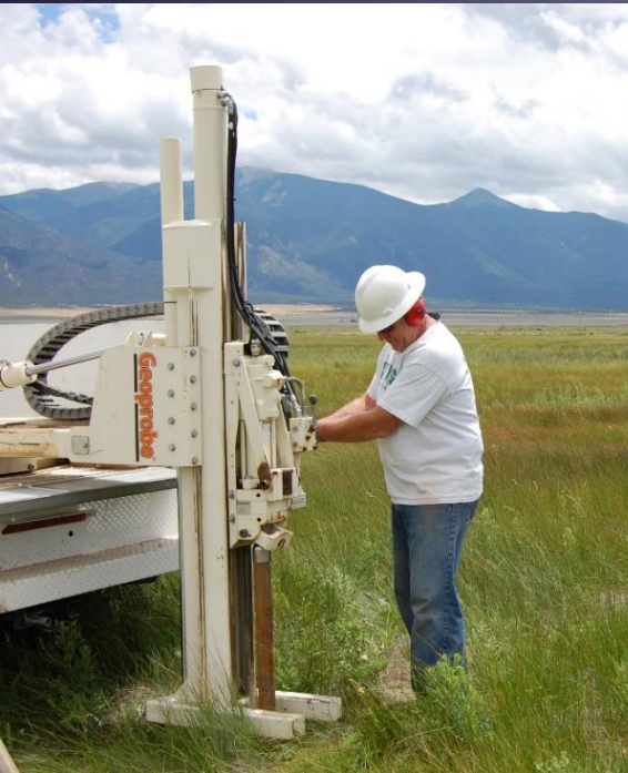
Hydrologic Technician Fred Gebhardt installing a piezometer using a truck-mounted Geoprobe, August 2016. Photograph by Amy Galanter, USGS.
