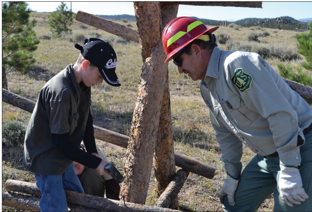
Figure 6 —Repairing a fence together on the Arapaho and Roosevelt National Forest and Grassland, Colorado (photo: USDA Forest Service)
