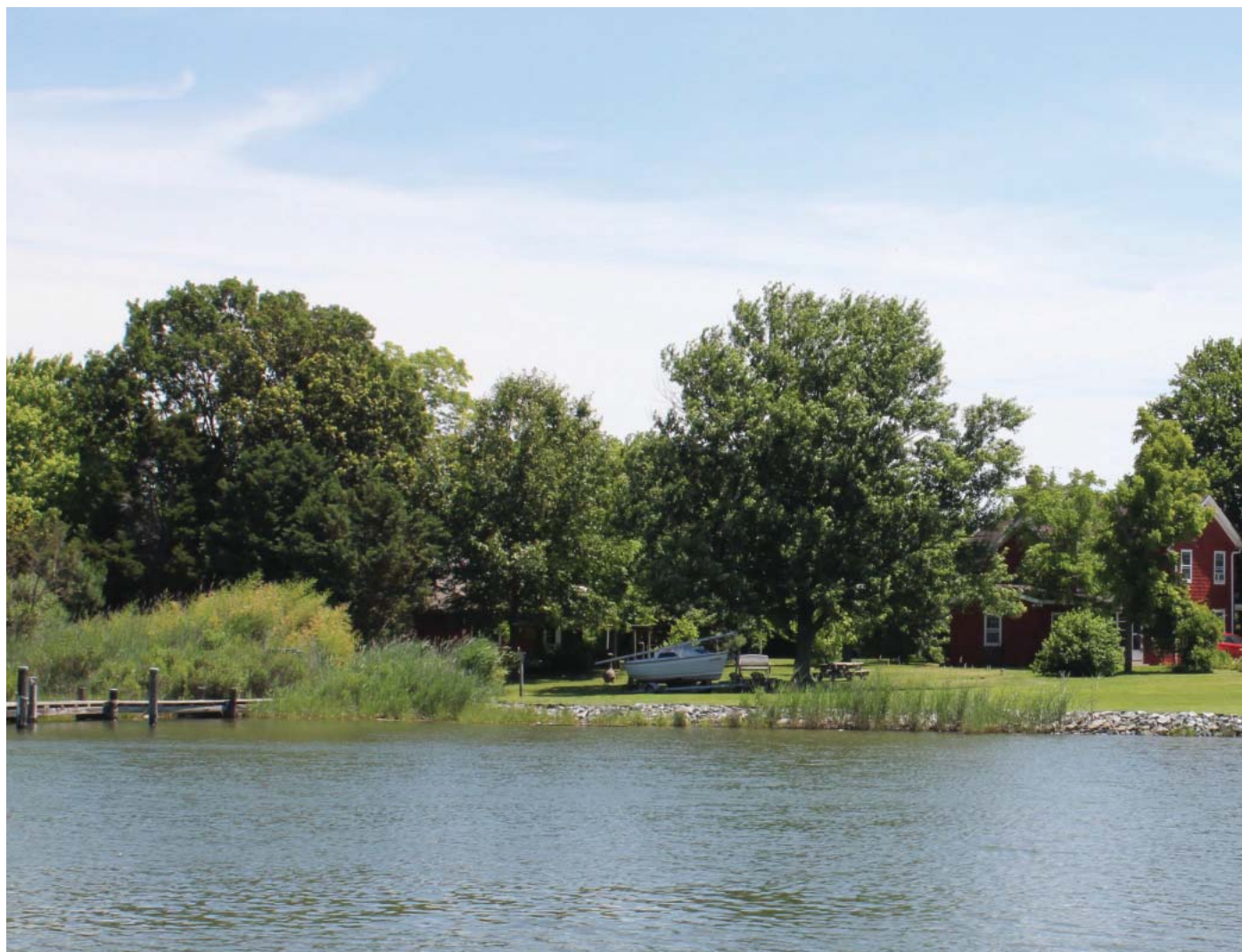
Riprap along Harris Creek. Photo credit: NOAA National Centers for Coastal Ocean Science
