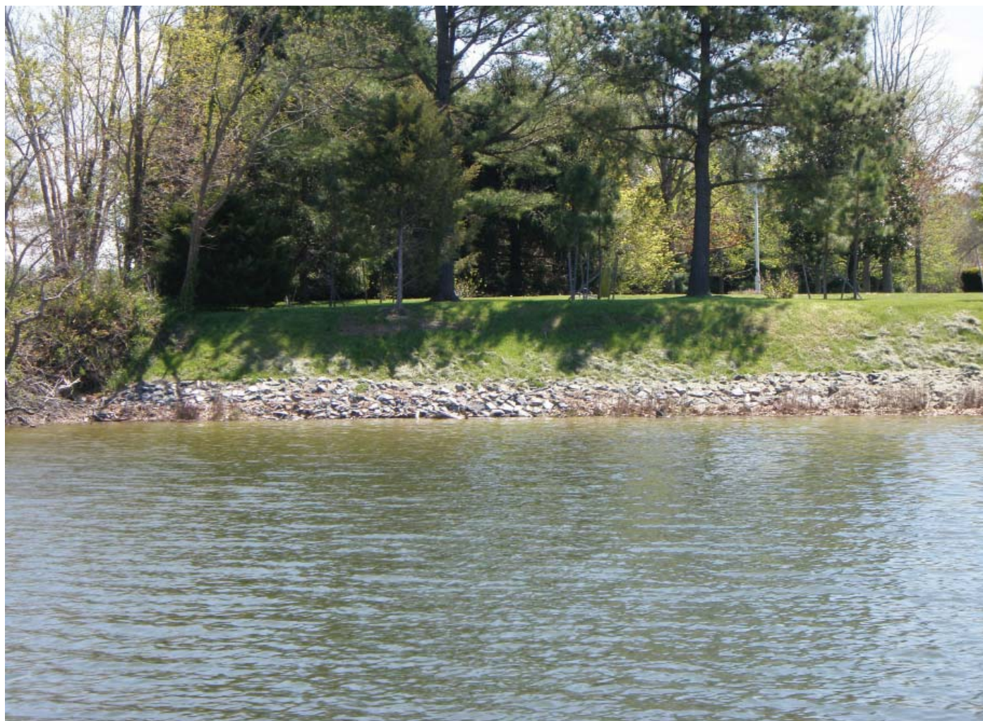
Riprap along the Tred Avon. Photo credit: NOAA National Centers for Coastal Ocean Science
